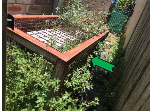
Photo 20. Exterior, north-west elevation, air conditioning unit – suspected ODS-containing unknown refrigerant gas.
