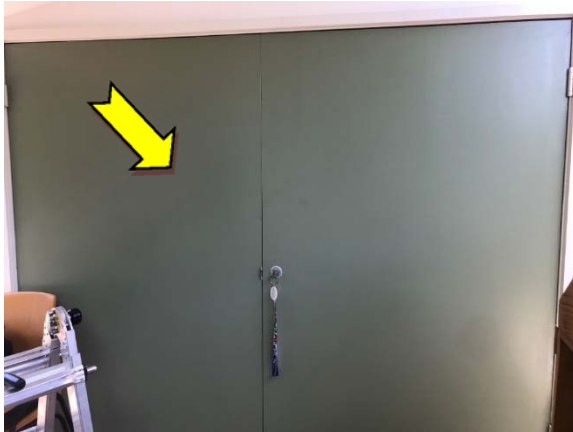
Photo 15. Exterior, doors and frames – suspected lead-containing green upper paint systems.
