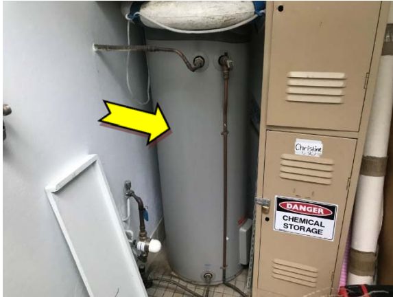
Photo 13. Interior, staff toilet, hot water heater – suspected SMF internal insulation material.
