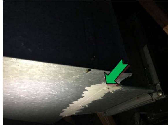
Photo 8. Interior, roof space, air conditioning ductwork – non asbestos-containing mastic sealant.
