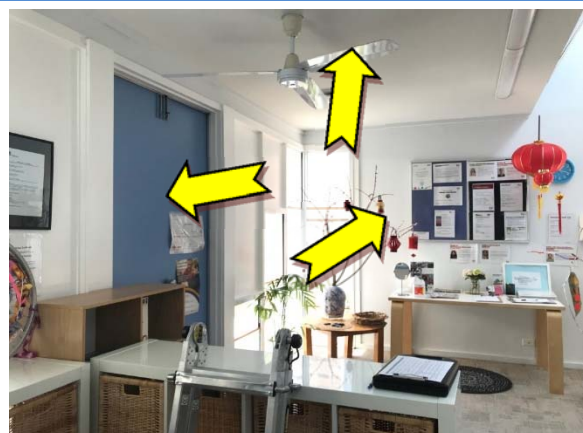
Photo 18. Interior, walls, ceiling and doors – suspected lead-containing white and light blued upper coloured paint systems.
