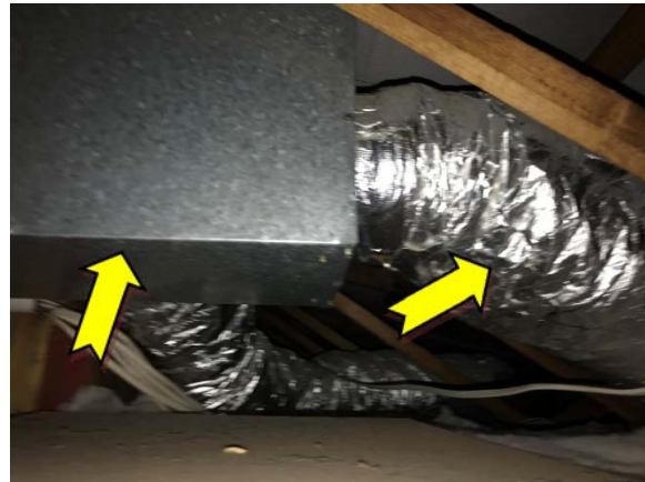
Photo 10. Interior, ceiling space, air conditioning ductwork – suspected SMF internal insulation.
