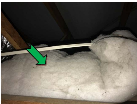
Photo 11. Interior, ceiling space, throughout – suspected non SMF insulation batts.
