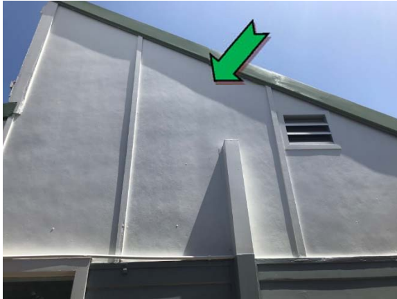
Photo 1. Exterior, north elevation, high level infill panels – non asbestos-containing fibre cement sheeting.
