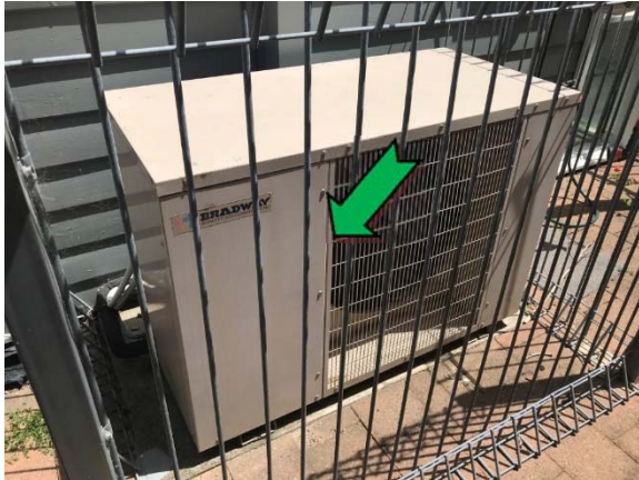
Photo 19. Exterior, north elevation, air conditioning unit – suspected ODS-containing unknown refrigerant gas.
