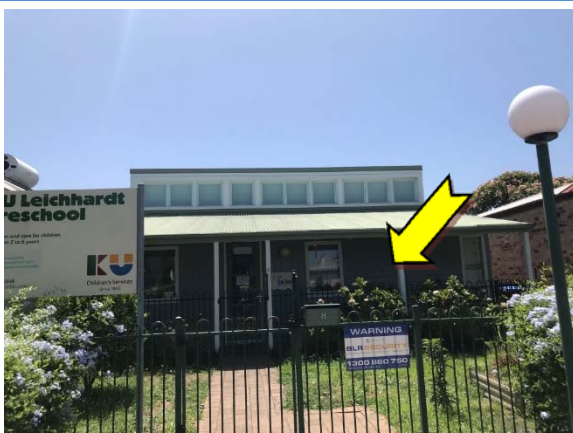
Photo 17. Exterior, walls, throughout – suspected lead-containing grey upper paint systems.
