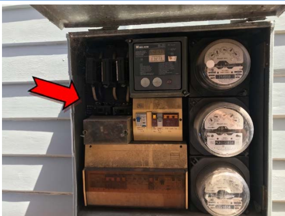
Photo 5. Exterior, north elevation, electrical backing board – suspected asbestos-containing bituminous backing board.
