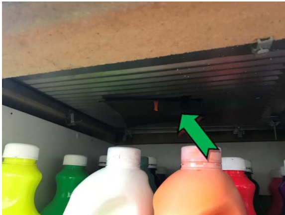
Photo 9. Interior, craft room, under sink, sink pad – assumed non asbestos-containing bituminous material.
